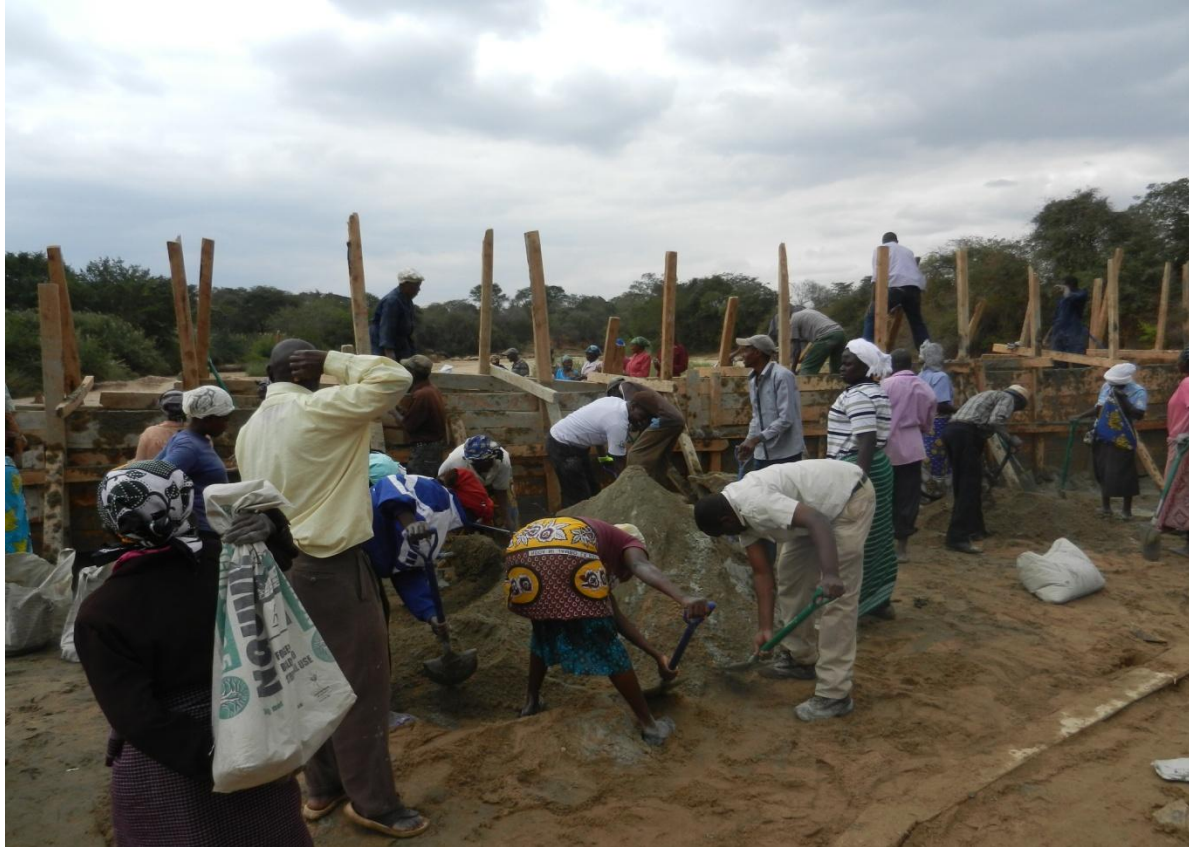
Figure 2: Mixing cement at the Kaiti River Self Help Group's sand dam extravaganza, July 2013.
