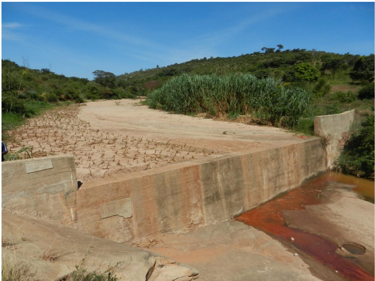
Figure 1: This sand dam was built in 2009 by the Kitandi Fruit Tree Growers SHG on the Kaiti River in Makuieni County. It was extended one year later to reach its present height. It has a 17.9 meter spillway and holds nearly 11,000 cubic meters of sand and 4,000 cubic meters of water when saturated. Note the strong stand of napier grass on the right stream bank. It is also planted as cuttings on the left bank. (Photo by the author, July 2013)
