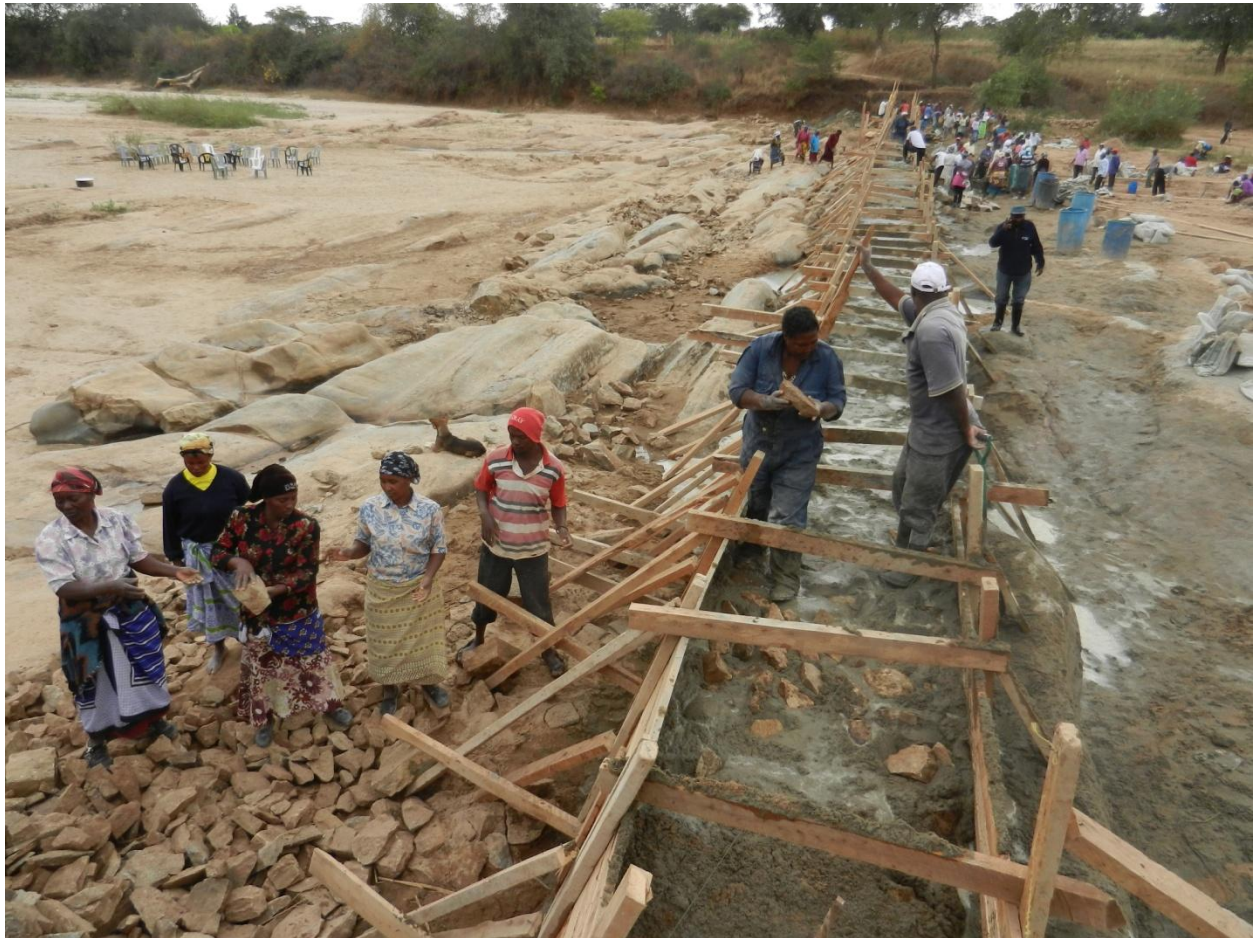
Figure 3: Adding rock to the cement mix near the end of the work day on the Kaiti River sand dam.
