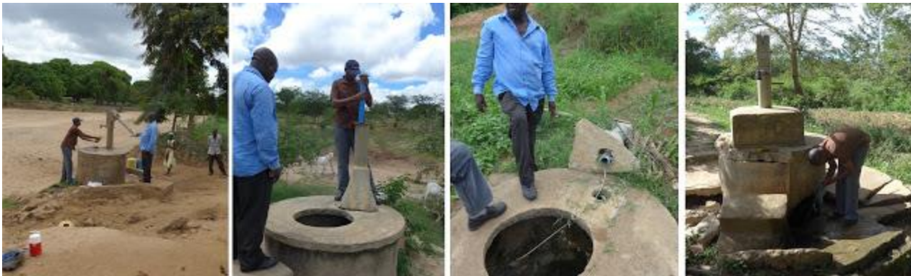
Fig. 22. Examples of pump wells. Pump well at left is functional, those to the right are broken from vandalism, floods, and general breakage.
