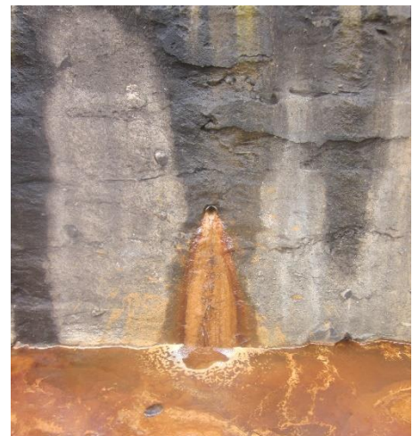
Fig 14. Pipe in face of dam structure draining water from deep sand, showing red color of water presumably from iron.
