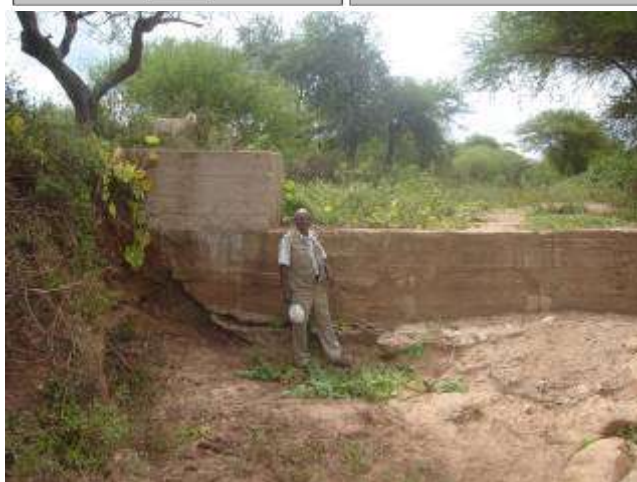
Erosion of left hand bank shows the foundation and apron do not extend into the riverbanks
