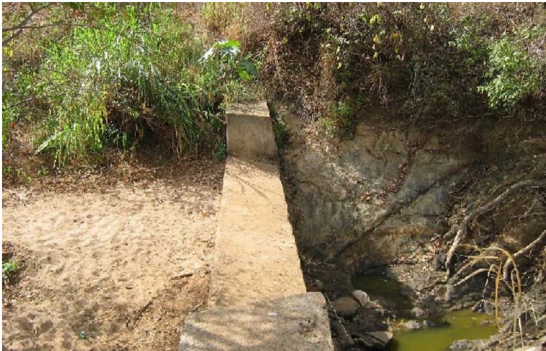
Figure 4. Example of a Sand Dam. The word 'sand' refers to storing water within the sand that accumulated behind the dam. A 'mature' dam is a dam where sand is accumulated to the highest level of the dam, hence generating the highest potential for water storage
